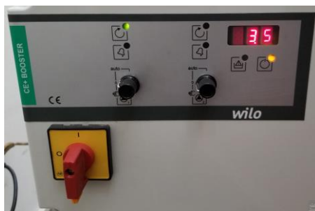
Fig. 9. Pump control panel
