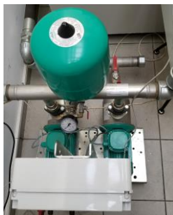
Fig. 8. The irrigation stand pumping group
