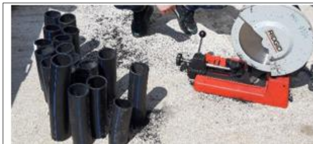
Figure 1. The pipes used for experimental study
