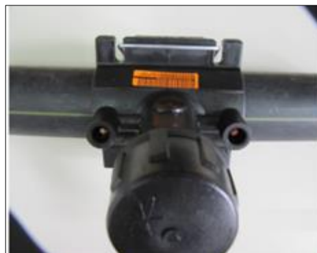
Figure 22. Welding the polyethylene tees to the PE 100 SDR 11 pipe Dn 63 in diameter
